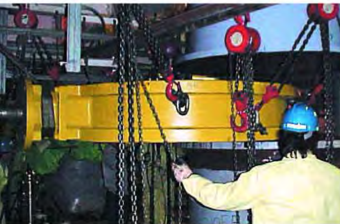
Installing a refurbished butterfly valve at Hope Creek Station. FTI assumes full ownership for its workscope related to valves, offering innovative risk-sharing and performance-based contract clauses.
