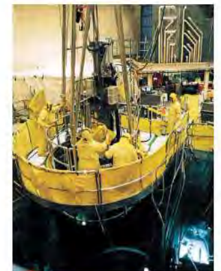
Framatome Technologies, teamed with Master Lee, won baffle bolt inspection and replacement contracts at all U.S. two-loop plants.
